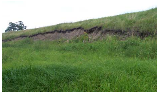
Figure 2.17 UNACCEPTABLE earthen embankment failure. (MN)
