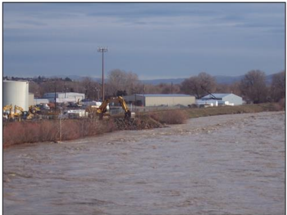
Rip-Rap Repair at NC Machinery Levee January 2009
